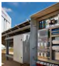
Pv Solar Test Lab
